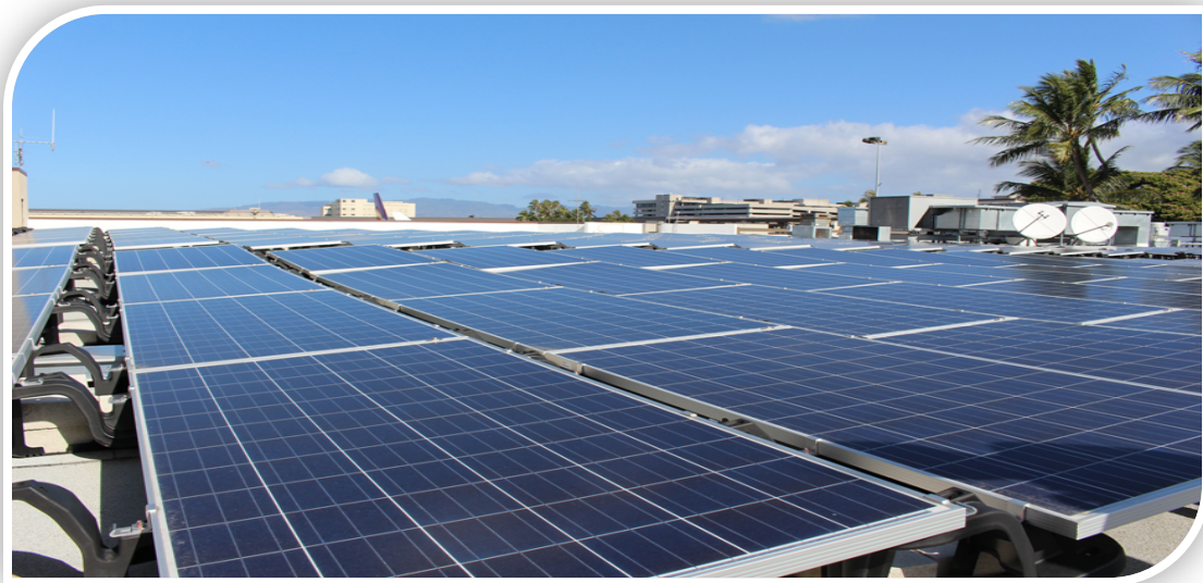
Above: Over 2,000 solar PV panels were installed in the 2 nd quarter of 2015, greatly reducing the energy purchased.
